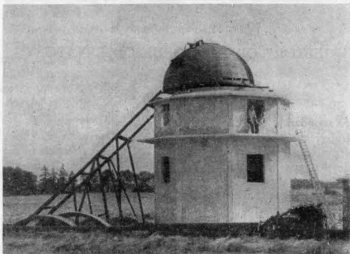
7. The erection of the first astronomical building in 1948 - the five meter dome constructed in Toruń, brought to Piweice and mounted on top of the building
