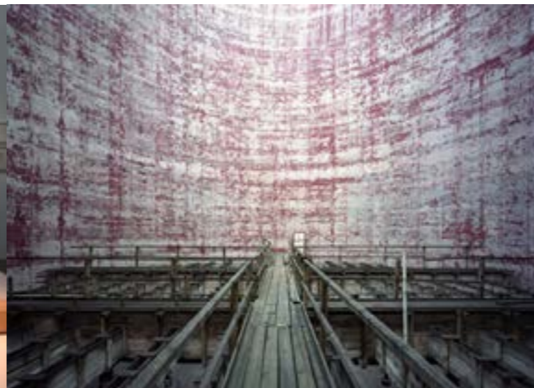
© Cooling Tower, Power Station, Scheibler Textile Factory, Łódź, 2012 / Yves Marchand & Romain Meffre / Polka Galerie
